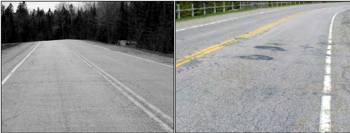
Figure 13. Highway 11B Typical Condition and Localized Plough Damage in 2011
