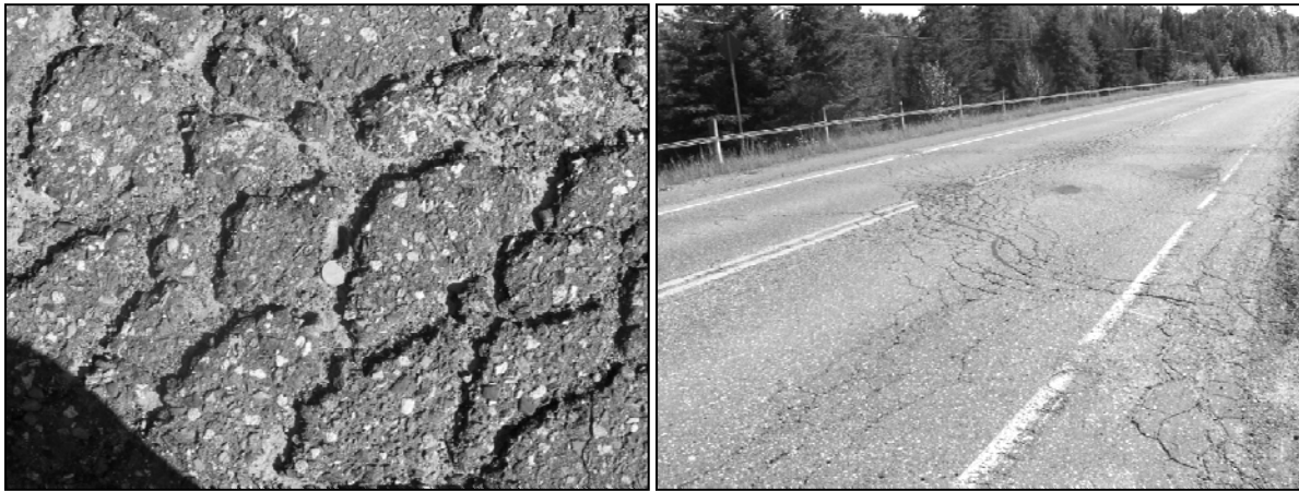
Figure 12. Wide-Spread Block Cracking on Highway 11B
