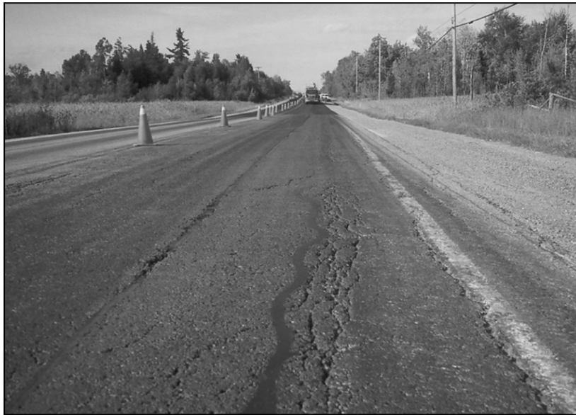
Figure 5. Condition of Original Roadway prior to Micro Surfacing on Highway 15
