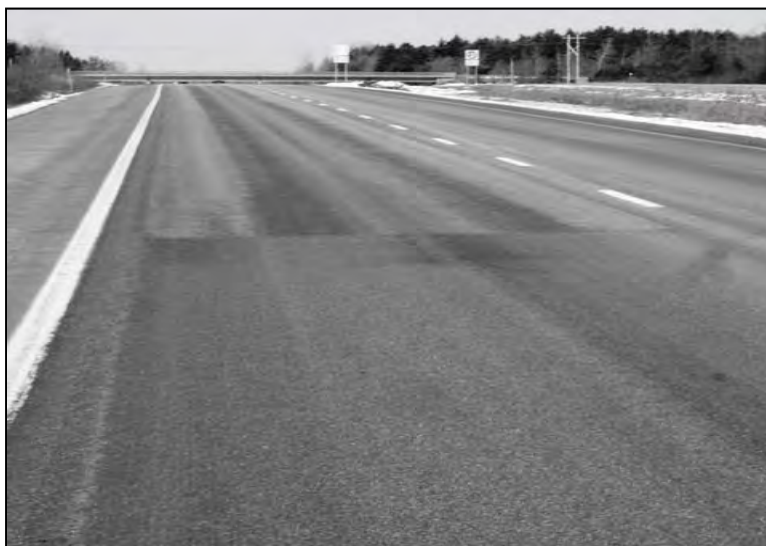
Figure 2. Illustration of the Effect of Excess Water on the Surface Characteristics
