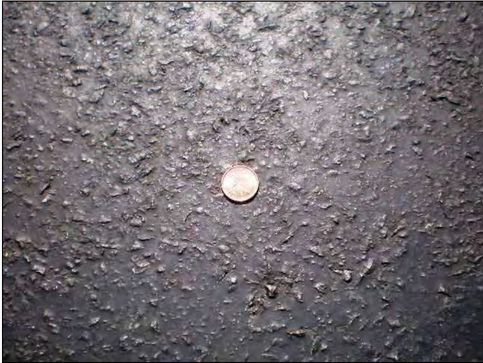
Figure 3. Micro Surfacing Macro Texture after Using Excess Water
