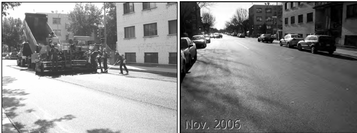
Figure 1: Warm Mix Placement on Rue Ball in August 2005 and One Year Later
