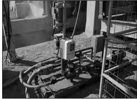
Figure 5b: Pump/Metering System
