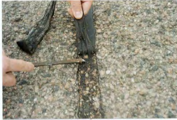
Figure 1. Crack Sealant Debonding on Highway 11, Southbound, Oro Road to Orillia, Summer 1999
