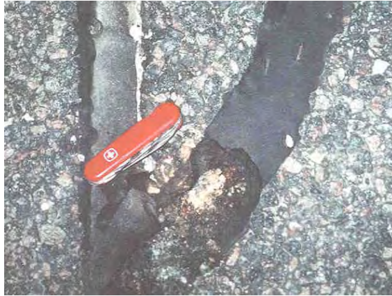
Figure 3. Sealed Longitudinal cracks on Highway 401, Westbound in Mississauga
