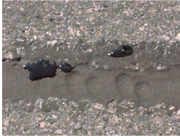
Figure 15. Water Forced out of a Sealed Transverse Crack on Runway 08-26 at Canadian Forces Base Goose Bay
