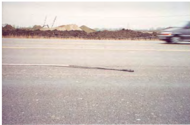
Figure 2. Failing Crack Sealant on Highway 50, Region of Peel, 2001
