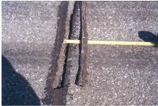
Figure 5. Debonded Crack Sealant in a Transverse Crack on Runway 08-26 at Canadian Forces Base Goose Bay
