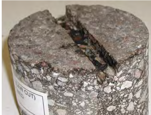
Figure 13. Partial Adhesion and Partial Cohesion Sealant Failure in a Wet, Pull-out Test with a Saw-Cut Reservoir
