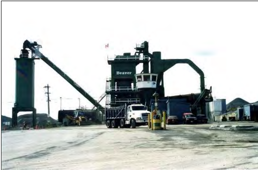
PHOTOGRAPH 2: Beaver Road Builders 8000 lb Barber Greene Batch Plant
