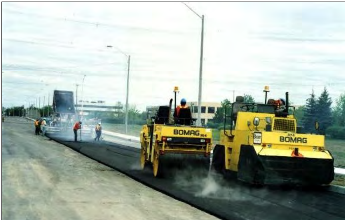
PHOTOGRAPH 4: Compaction Equipment Rolling Hot Mat. Note Heating Vent and Skirts on Rubber Tired Roller to Aid in the Prevention of Pick-up.
