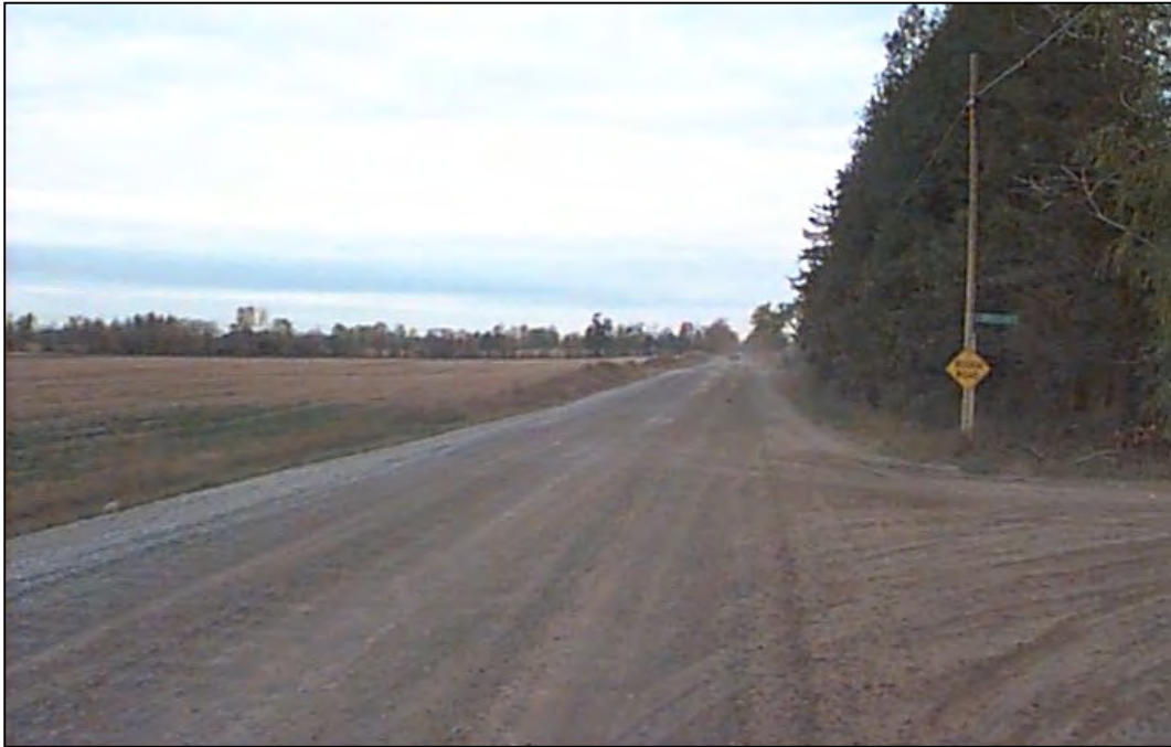
Figure 1 – Condition of York/Durham Line 30 before Pavement Rehabilitation
