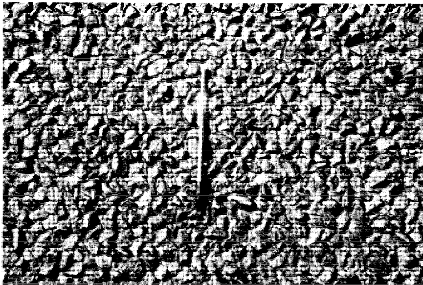
Fig. 5. Close-Up of Surface Treatment Shown in Figure 4.
