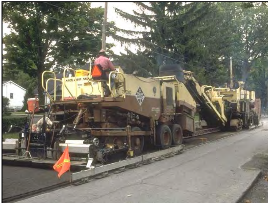
Photograph 3: Two-unit recycling train
