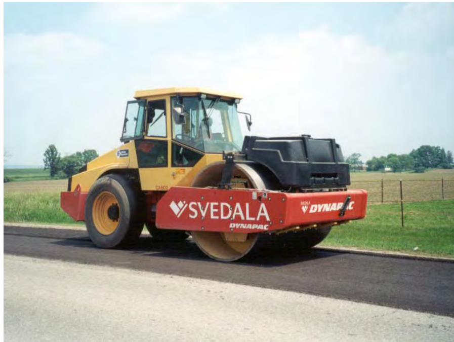
Photograph 8: Modified large single drum vibratory roller fitted to compact cold recycled material
